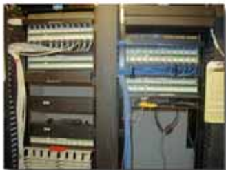
Patch Panel Terminations
