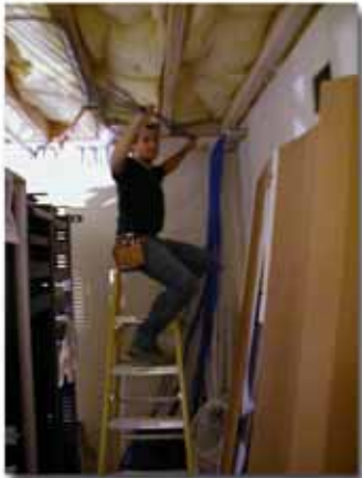
Cable & Fiber Routed
